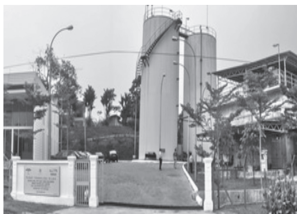
Figure 4. A zero discharge palm oil mill effluent treatment pilot plant at the MPOB's Experimental Palm Oil Mill (POMTEC), Labu.
