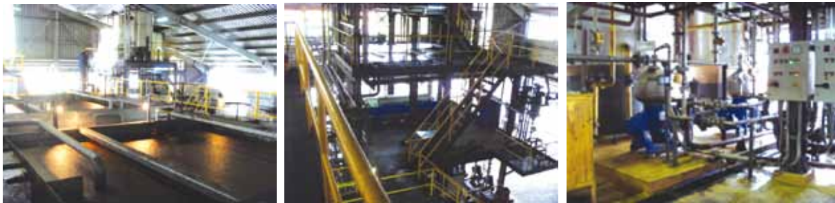
Figure 2. Coalescing clarifier (OILSEP) at Vichitbhan oil mill – second generation.
