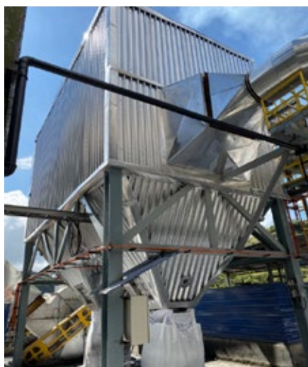
Figure 9. Hot gas filtration on 40TPD municipal solid waste incineration plant.
