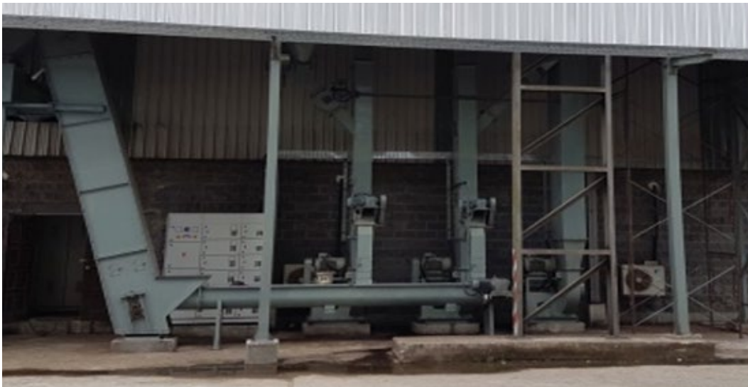
Figure 15. Pre-cleaning system installed at the Sime Darby Kernel Crushing Plant, Carey Island, Banting, Selangor.
